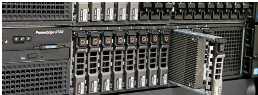
Dell end-to-end solution consisting of PowerEdge, EqualLogic, S-series & N-series Networking and SonicWALL.
